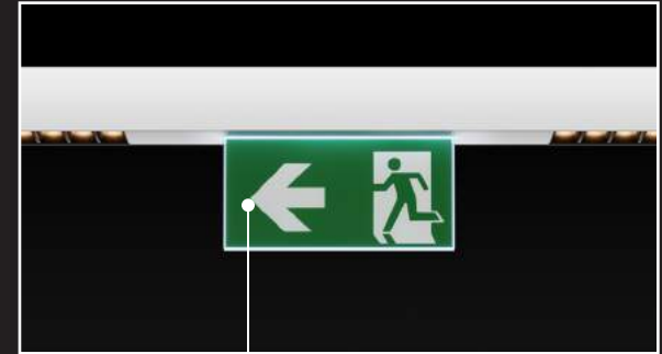
INTEGRATED EMERGENCY SIGNAGE
